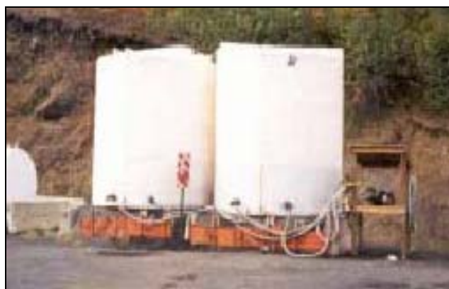
Idaho DOT Chemical Storage Tanks
